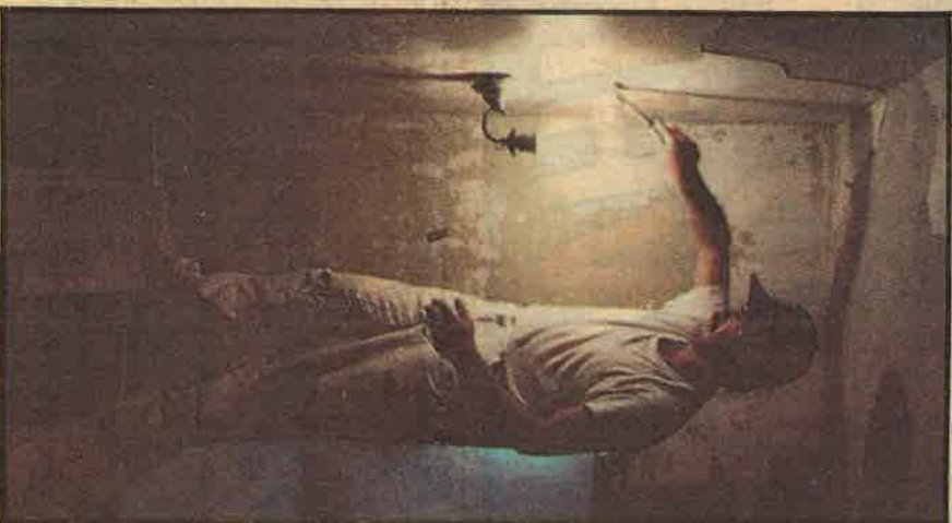
Ray Taylor of Detroit repairs plaster in the mansion. Owner Michael Allen estimates renovations will total $1.2 million.
