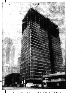
Construction of the new Detroit Bank and Trust Building on Fort Street at Washington Boulevard is progressing steadily. Pictured above is the building as it looked during the last week of 1962.
