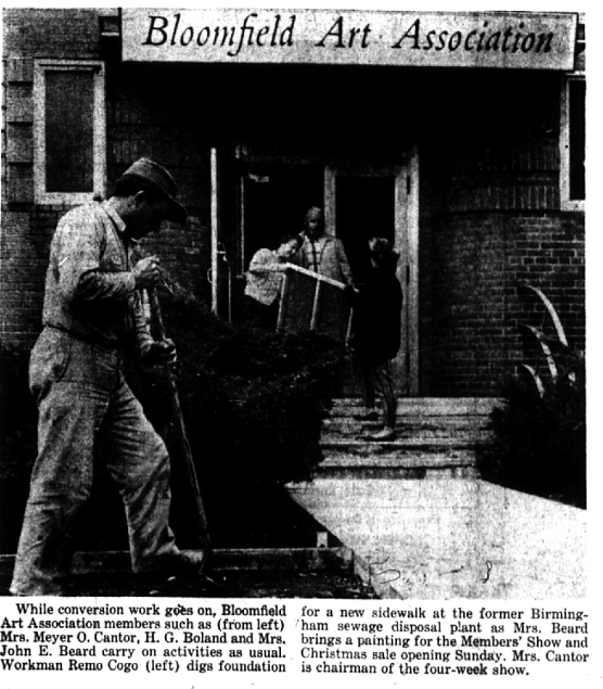
While conversion work goes on, Bloomfield Art Association members such as (from left) Mrs. Meyer O. Cantor, H. G. Boland and Mrs. John E. Beard carry on activities as usual. Workman Remo Cogo (left) digs foundation for a new sidewalk at the former Birmingham sewage disposal plant as Mrs. Beard brings a painting for the Members' Show and Mrs. Cantor is chairman of the four-week show.
