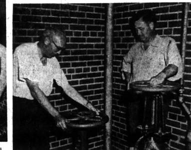
WATER FROM SOC Water Authority poured into Birmingham in June. Here Director L. R. Gare, turns the valve which sends water coursing into Birmingham pipes as Bob Rothe, representing the authority's consulting engineers, watches.
