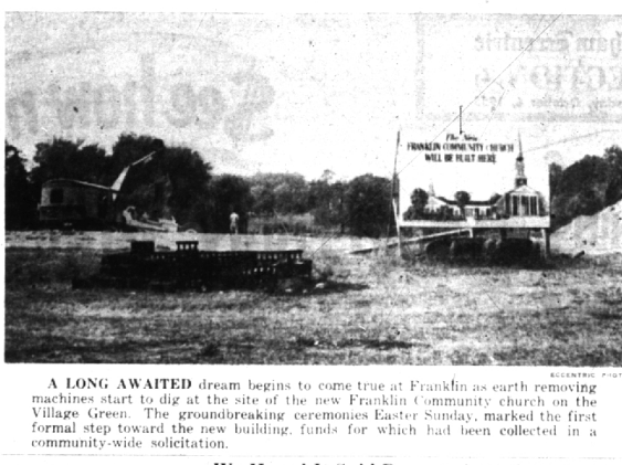
A LONG AWAITED dream begins to come true at Franklin as earth removing machines start to dig at the site of the new Franklin Community church on the Village Green. The groundbreaking ceremonies Easter Sunday, marked the first formal step toward the new building, funerals for which had been collected in a community-wide solicitation.
