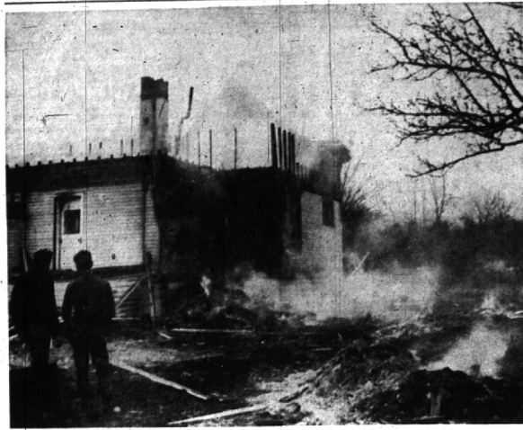
WHILE THE HOUSE-WRECKERS ate luncheon, fire gave them an assist and burned away a section of this old house being torn down on N. Hunter Blvd. Russ Brant, head of the wrecking crew, said splinter pieces of the wood were being burned on the property when the dried grass caught fire and spread to the house. The crew was eating lunch at a nearby restaurant at the time. Birmingham firemen answered the original call, but returned when Bloomfield township fighters appeared. Owner of the house, J. W. Jenkins, 1716 W. Outer Drive in Detroit, gave Bloomfield township firemen a "no damage" claim since it was being demolished. (Eccentric Photo)
