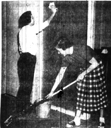
JUNIOR LEAGUERS Mrs. James Joyce polishes the new glass door, separating two doctors' rooms in the future clinic at 300 East Maple while Mrs. Steele Sellers energetically uses the mop. Many members are working on the clinic project and soon will have the decorating completed.
