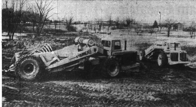
HEAVY EQUIPMENT RUMBLES over the site of the planned new Bloomfield Hills high school at W. Long Lake and Andover roads as rough grading operations proceed in preparation for construction. Twenty-four of the 32 acres that comprise the site were donated to the Bloomfield Hills
