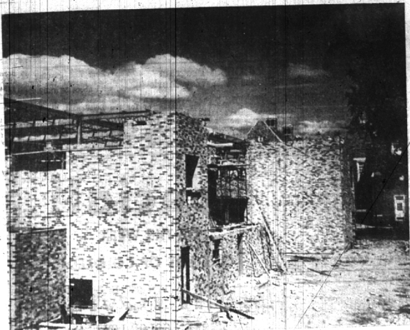
QUARTON SCHOOL ADDITION NEAREST TO COMPLETION Six classrooms will ease school population growth (Eccentric Staff Photo)
