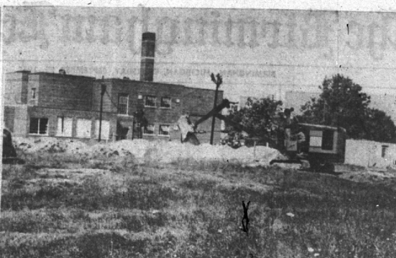
THE SOUTHFIELD SCHOOL DISTRICT is in the midst of a building pinch common to all suburban Detroit developments. To temporarily relieve the crowded situation at Southfield school, Ten Mile and Berg, an eight-room addition is under construction. Diggers and graders are pushing work schedules to complete as much of the work as possible before bad weather sets in. The new structure will house two kindergarten rooms and other oversize classrooms. The present addition and future enlargements. The building will be of cinder block and brick. (Eccentric Staff Photo)
