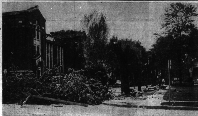
TREES ALONG W. MAPLE ARE REMOVED TO PERMIT STREET WIDENING From this angle, trees used to hide side of Baldwin elementary school, now exposed.
