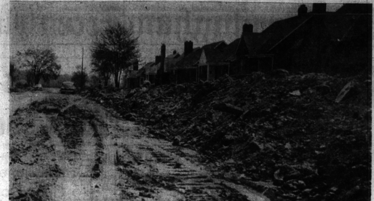
WHO'S GOING TO CLEAN UP THIS MESS? This question baffles both the city and the Taylor Brothers Construction company, paving contractors preparing to pave Manchester between St. Andrews and Coalgate. The paving firm has been confronted with mounds of earth, building debris and gravel on other streets to be paved and has taken the time to clear the rubble before laying the concrete. Taylor Brothers now feel that the city should force the home builders to clean up the trash before the company is asked to improve the street. (Eccentric Staff Photo)
