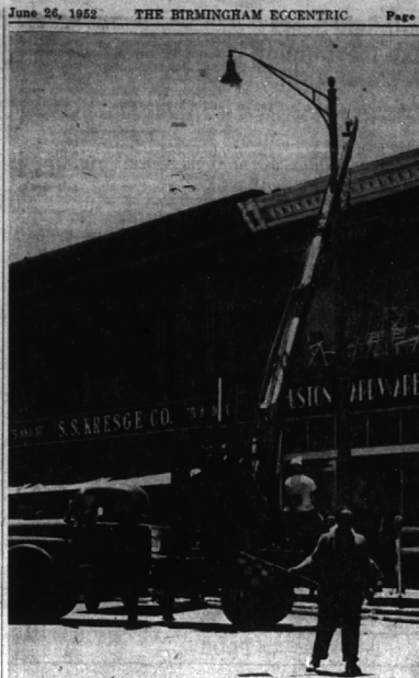
DETROIT EDISON EMPLOYEES INSTALLING one of two additional light poles on Woodward between Maple and Willits to brighten up the business section. The new lamps are higher and afford a greater radius of light. (Eccentric Staff Photo)
