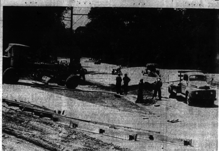
WORKMEN TACKLE THE CLEAN-UP JOB ON THE NEW W. MAPLE PAVEMENT Lincoln avenue detour is a thing of the past as main east-west artery is reopened. (Eccentric Staff Photo)
