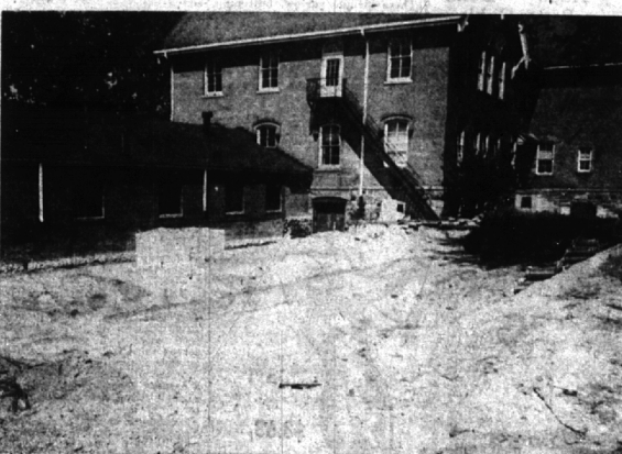
ALSO AT HILL school, this particular "hole in the ground" will eventually turn into a loading dock for trucks delivering school supplies. The program will call for the relocation of one door in the building which will give entry to a storage section for books and classroom materials for the several elementary schools in the Birmingham district. (Eccentric Staff Photos)
