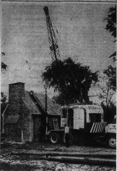
FIRE CHIEF VERN GRIFFITH , in white shirt alongside the crane, supervises the handling of new pipe lengths to deepen city's east well at Derby and Pembroke. The building is so constructed that a portion of the roof and back wall can be removed for major repair work. Iron-oxide pipes in the foreground have been taken from the well and will be cleaned for re-use. Capacity of the pump has been dropping off, so the city deepened the well to gain maximum supply through the summer.
