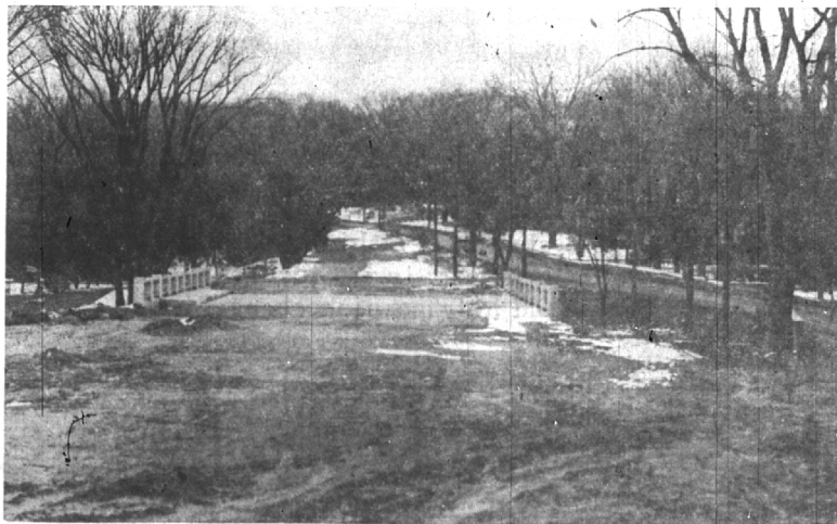
ALTHOUGH WHEN this picture was taken the approaches to the new $35,000 West Maple bridge looked pretty "rural", city officials assured motorists that it would not be much longer before the bridge was in use.
