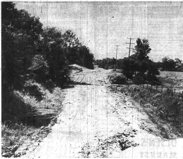
AS THIS PICTURE SHOWS, THERE IS A tremendous amount of work yet to be completed on Sixteen-Mile road between Adams and Woodward before motorists are able to use the new right-of-way. But the County Road Commission guessed that the new road may be opened in another month if weather, materials and labor conditions are favorable. The Sixteen-
