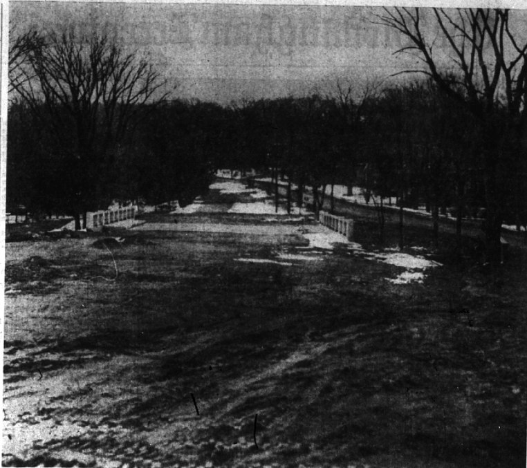
IT SHOULDN'T BE LONG NOW before motorists will be able to use this new $35,000 city bridge on West Maple over the River Rouge. Here's how it would look this week to a west-bound motorist. The old bridge and right-of-way is to the extreme right. The new right-of-way goes thru the center of the photo. At the extreme left center can be seen some of the tree trunks that were cut down last week to enable the paving contractor to put in the stretch west of the bridge. The contractor is expected to start construction late this month or early in May.
