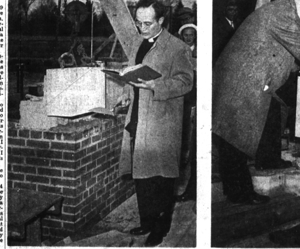
CORNERSTONES were laid Sunday for two new Birmingham churches. Pictured at the left is Rev. H. G. Allward, pastor of Our Shepherd Lutheran church, reads appropriate scriptural passages, at the ceremony, following the morning worship service. The $75,000 building will be the first of three units to be built on the 14 Mile road site east of Woodward. It is expected the building will be completed and ready for dedication in September. At 4 p.m., the cornerstone was laid for the new Methodist church on West Maple. Shown in the photo to the right, the Rev. Dr. Arnold F. Runkel places mortar for the stone after the corners of the 1871 cornerstone were added to items of current history. Various church officials took part in the ceremony with an address by Bishop Marshall Reed of the Detroit area.
