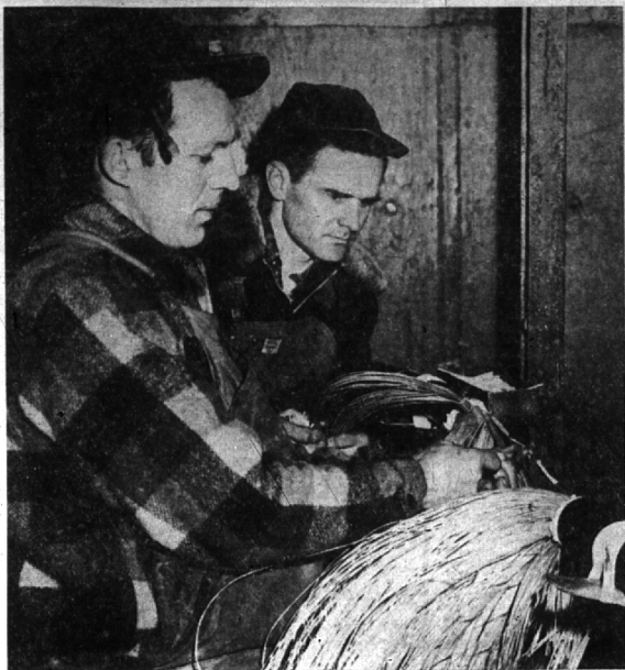
JOE SKIBA (LEFT) AND HELPER JOE VERESH SPLICE CABLES 4,200 individual phone wires involved in their job.
