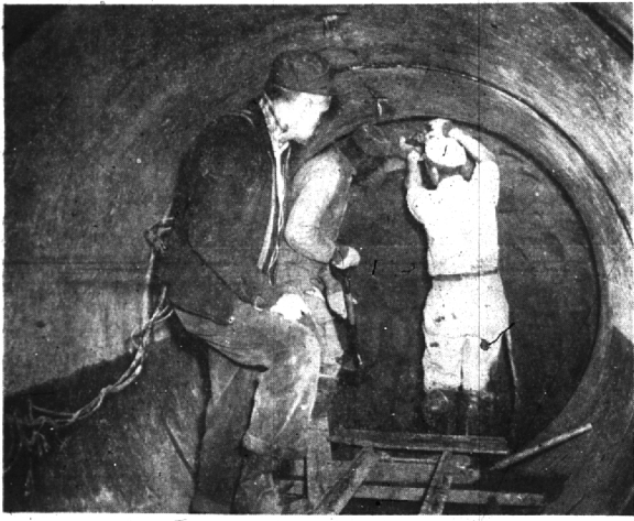
A sewer construction crew worked 50 feet under the Grand Trunk railway tracks last spring, putting in the new Webster relief sewer. By the installation of this sewer, homes in the eastern edge of the city were benefited.
