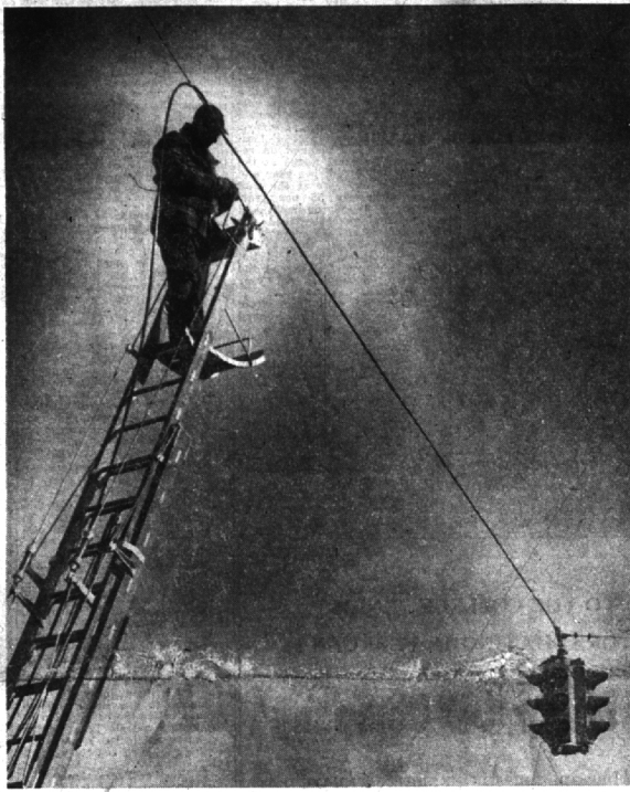
A member of the State Highway Department crew works on the installation of the new Woodward-14 Mile traffic signals, one of which can be seen at the lower right. The signals went up and were operating Dec. 14.
