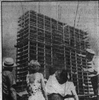
FRAMEWORK C. F. PEACE—Onlookers gaze at the progress being made on the new United Nations building in New York City. In the background is the skeleton of the U. N. Secretariat building, the first and tallest on the site. This 39-story structure will have 2700 air-conditioned offices.
