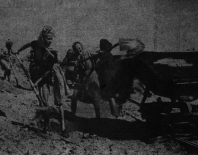
German women laborers shovel dirt into a rail dump car in clearing of the new airfield which the U. S. Army is building in the French sector of Berlin. The Army hopes to complete the field by winter to bolster the Berlin airlift. Photo by NEA-Acme staff correspondent Al Cocking.
