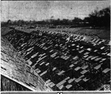
Five acres of flowers were ruined when the glass in these greenhouses at New Albany, Ind., was shattered by a 12-minute barrage of hail which tore the roofs off factories, dwellings and automobiles, entailing a damage of $500,000. Some of the stones were as large as baseballs.
