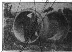
Enormous stocks of the Bloomfield Village Drain, now going underground. The taller man is 6 feet 2 inches. To the rear is one of five ditching machines now working at Bloomfield Village. The drains are scheduled for completion November 1st.
