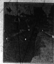
Installation of the huge sewer and water systems, now under way at Bloomfield Village, is personally supervised by C. W. Hubbell, nationally known engineering expert and former engineer for the City of Detroit.
